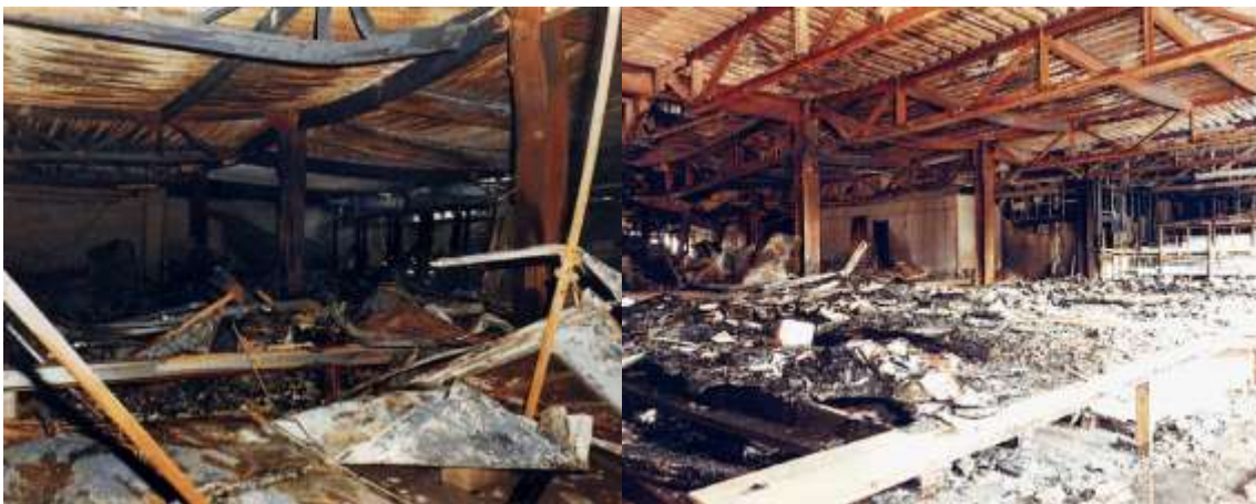
Figure 1. Fire damage to a building frame. Extracted from SCI P113 Investigation of Broadgate Phase 8 Fire [4].
