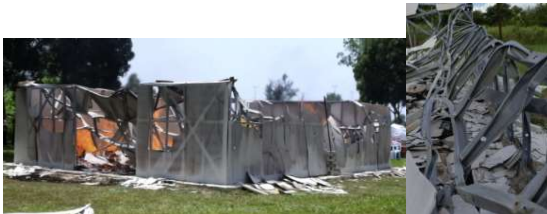
Figure 2. Building failure from a fire. Extracted from Roy et al. [5].
