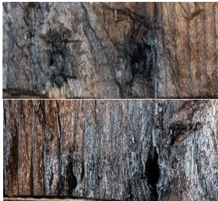
Figure 35. Pictures of the jointed area showing marks from the mechanical fasteners, Test 2 using nails (upper picture), and Test 3 using screws (bottom picture)
