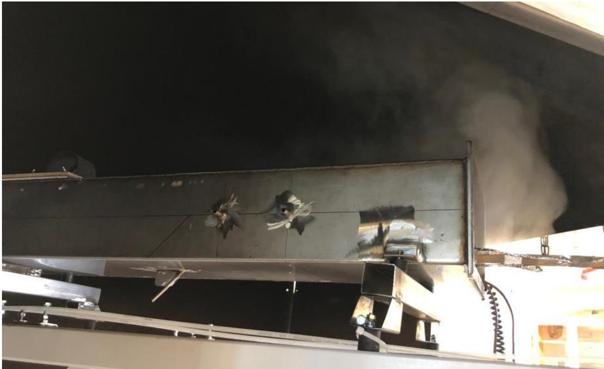
Figure 15 Smoke thickness formation at duct outlet
