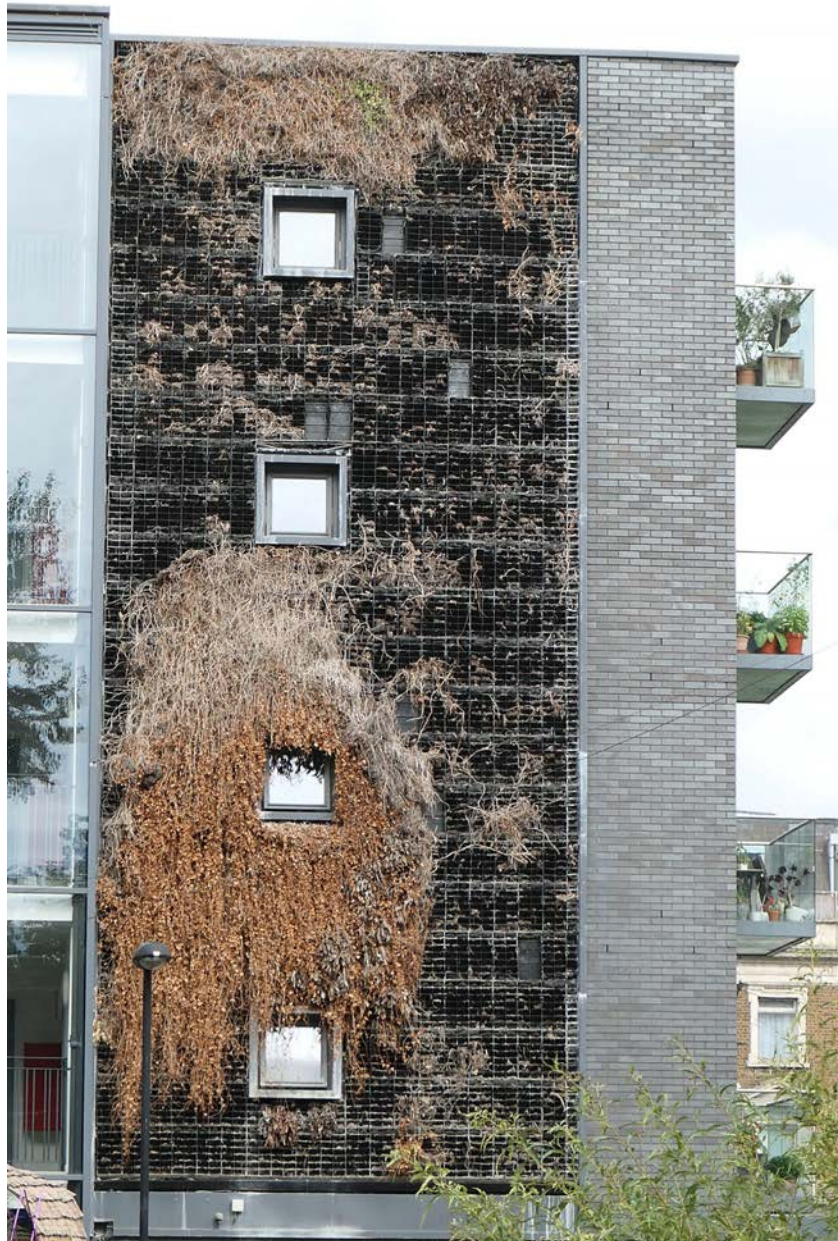
Figure 1: Decaying Green Wall (Pearman, 2021)
